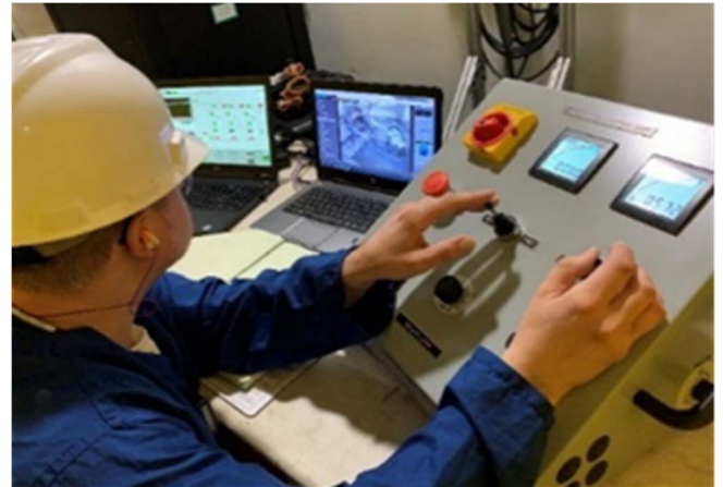
Undervessel sump cleaning control station
