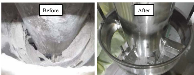
Radwaste encapsulation system cleaning
