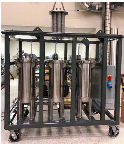
AMFM-S300 skid-mounted filtration system
