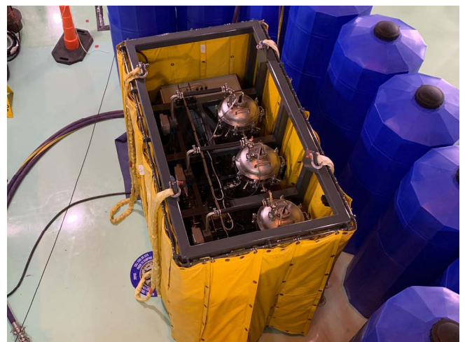
AMFM-S300 filter system used during cleaning
